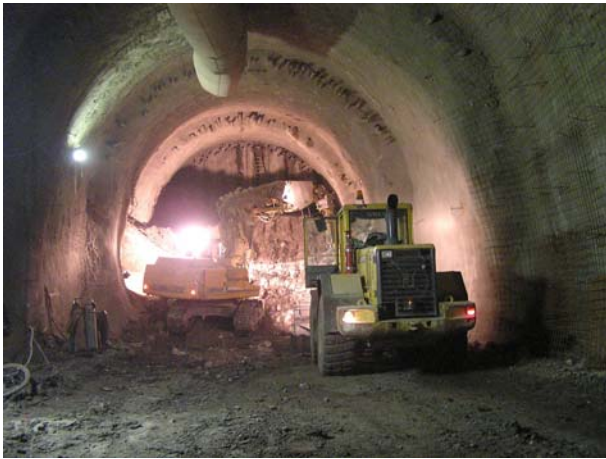
Fig. 11: Tunnel construction under micropile umbrellas the horizontal jet grouting columns (to increase their stiffness), but like the jet grouting columns drilled into the face, this approach was finished after the third section.
