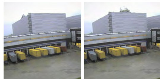
FIGURE 2. Pictures from a security camera taken during the storm in 2013, the roof failure is visible.
