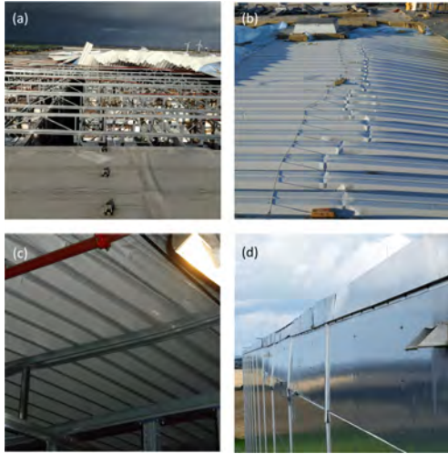
FIGURE 3. Qualitative description of typical damages: (a) Partically opened roof, (b) buckled sheets, (c) bent girder and (d) deformed parapet.
