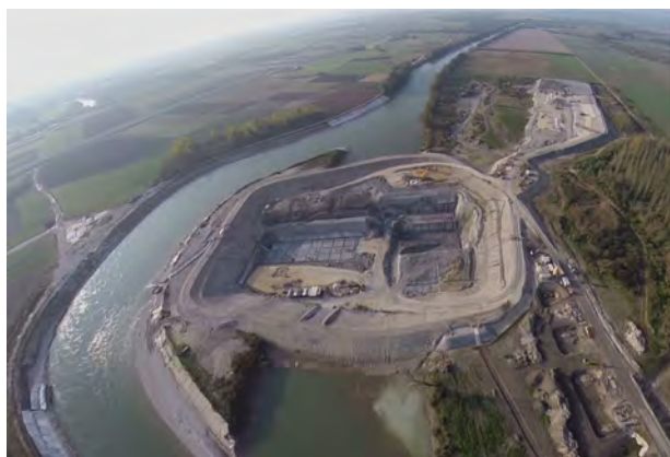
FIGURE 21. A view to the temporary dike, constructed from soil mixture and used as part of the large scale test embankment.
