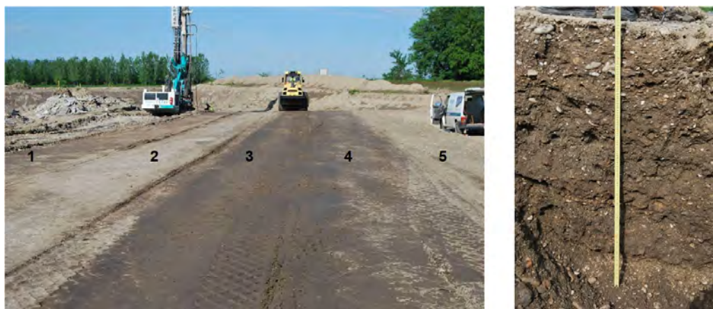
FIGURE 20. Vibratory roller during compaction on one of the test fields (left) and a view to the control pit in one of the test layers (right).
