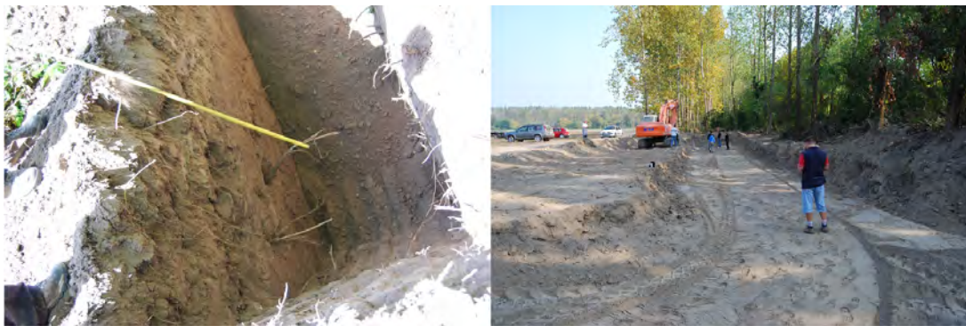
FIGURE 9. Depth of the roots (left) and the size of the first of four test fields prepared to study the roller compaction efficiency (right).
