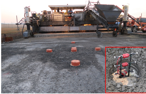
FIGURE 2. Vibrating wire gauges under protective covers. Detail at one assembled location.
