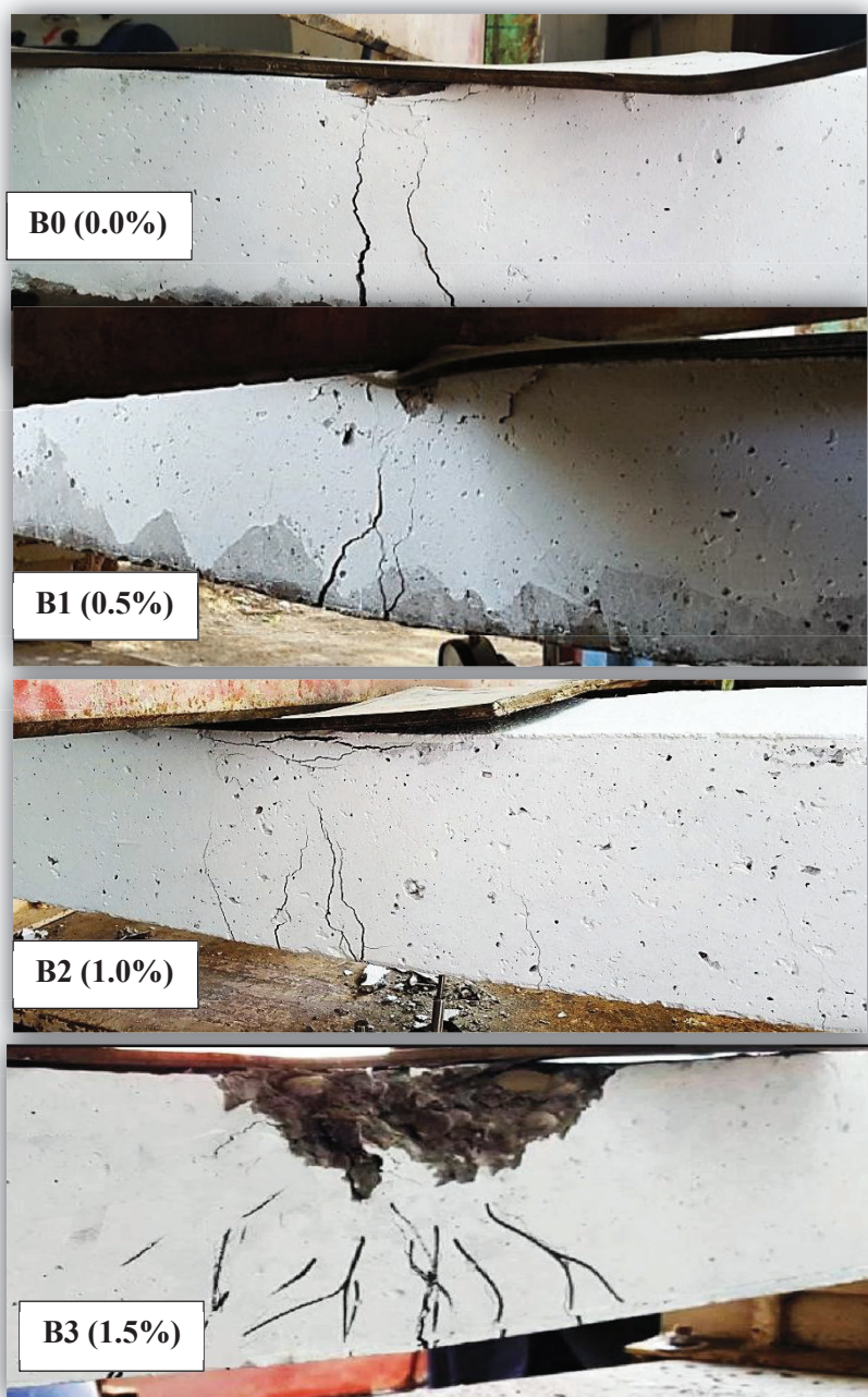
Figure 5: Failure mode of reinforced concrete tested beams
