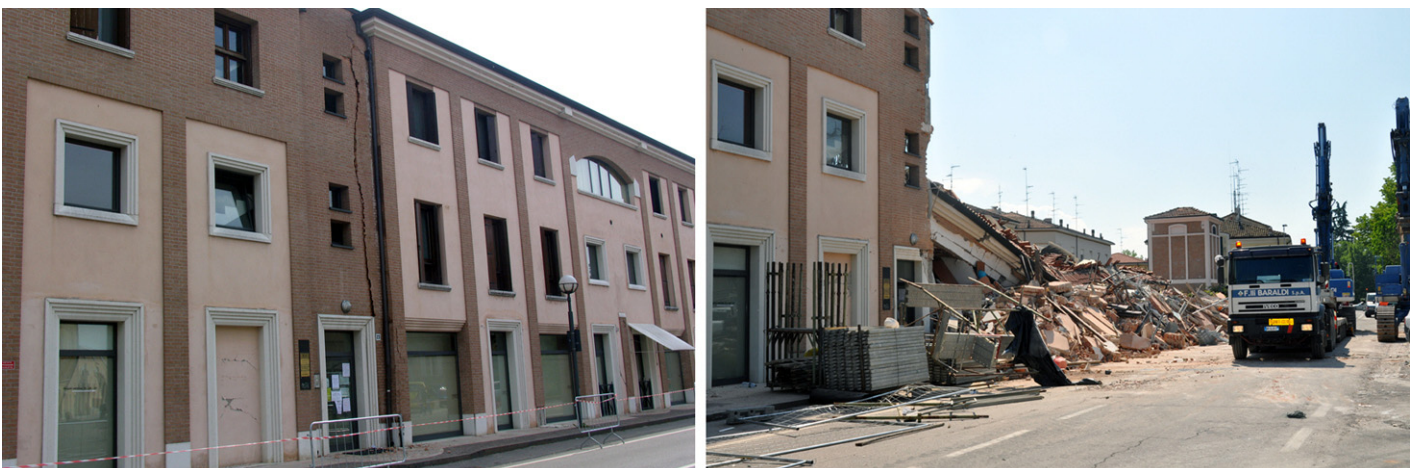
Figure 4. Increase in the damage to reinforced-concrete buildings, for May 20, 2012 (left), and May 29, 2012 (right), in Cavezzo.
