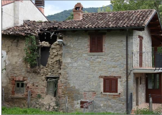
Figure 2: Pascellata (Valle Castellana): masonry building with walls faced with stone and rubble masonry fill. The part in bad state of maintenance compromises the rest of the building.
