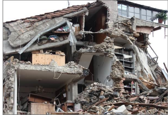
Figure 3: Amatrice: retrofit with (reinforced) concrete slab on old vertical walls without adequate reinforcement or proper connections between walls and floor.
