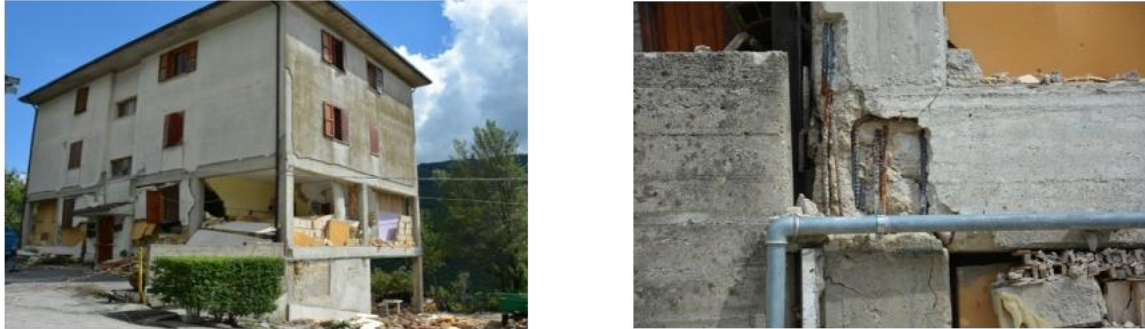
Figure 3: a) Reinforced concrete building in Pescara del Tronto, b) Detail of the damage to a beam-column joint.
