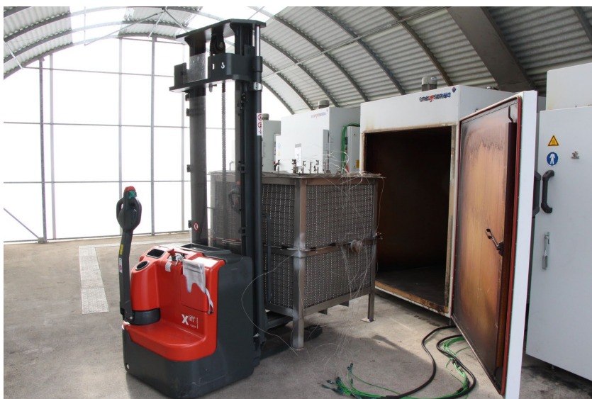
Figure 1: Weather protection tunnel with 4 ovens and equipped sample container (1,000 dm 3 ) with petroleum coke sample
