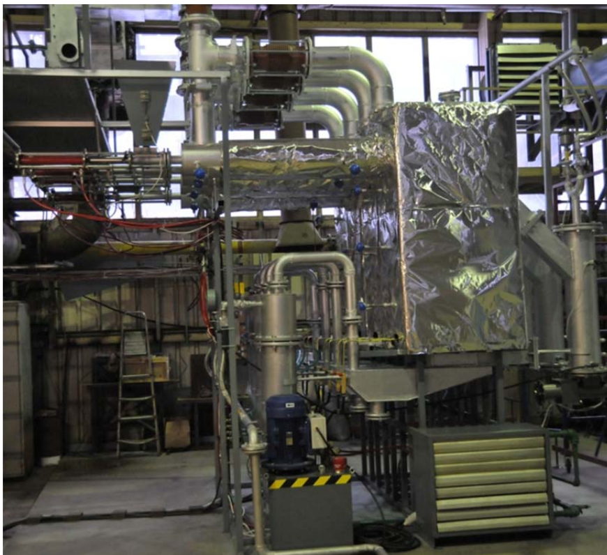
Figure 5: The setup of two-stage pyrolytic conversion technology of biomass into a gaseous fuel (electric power is 50 kW).
