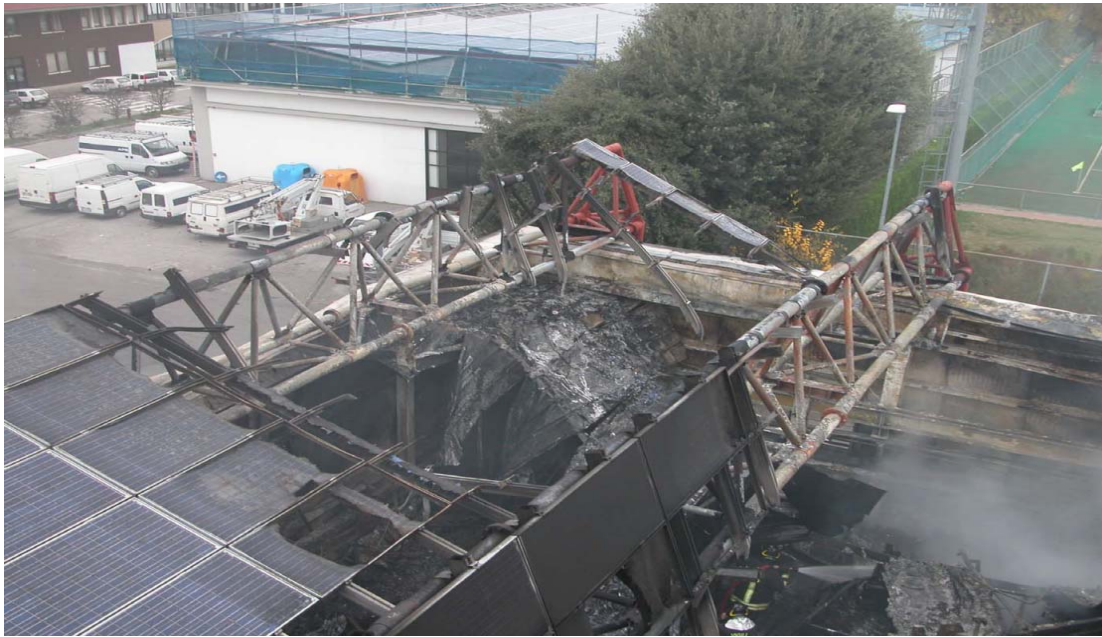
Figure 2: a 1000 sq meters warehouse housing a PV plant keep on fire. The evidence of the fire investigation conducted reported various elements in charge of PV Plant.
