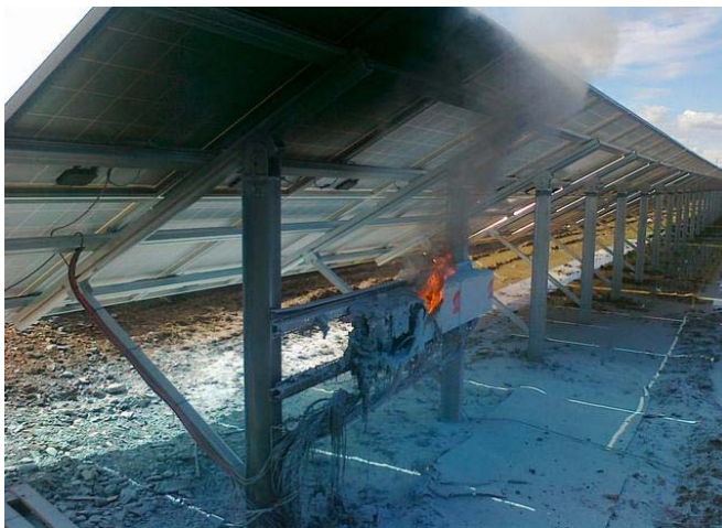
Figure 3: the Fire of a Connection Box in a ground PV Plant.
