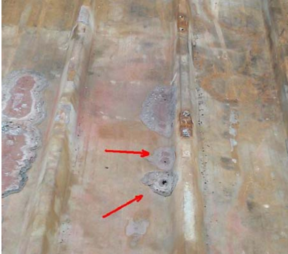
Figure 4: the The DC arcing effects on a external side of a polyurethane sandwich.
