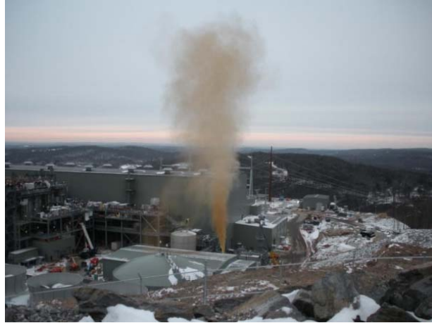
Figure 1: Cleaning of fuel gas piping by gas blow at Kleen Energy site one week before incident (CSB, 2010).
