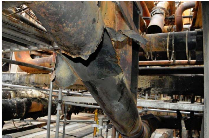
Figure 3: Pipeline degradation due to sulfidation corrosion at Chevron Richmond refinery (CSB, 2013).
