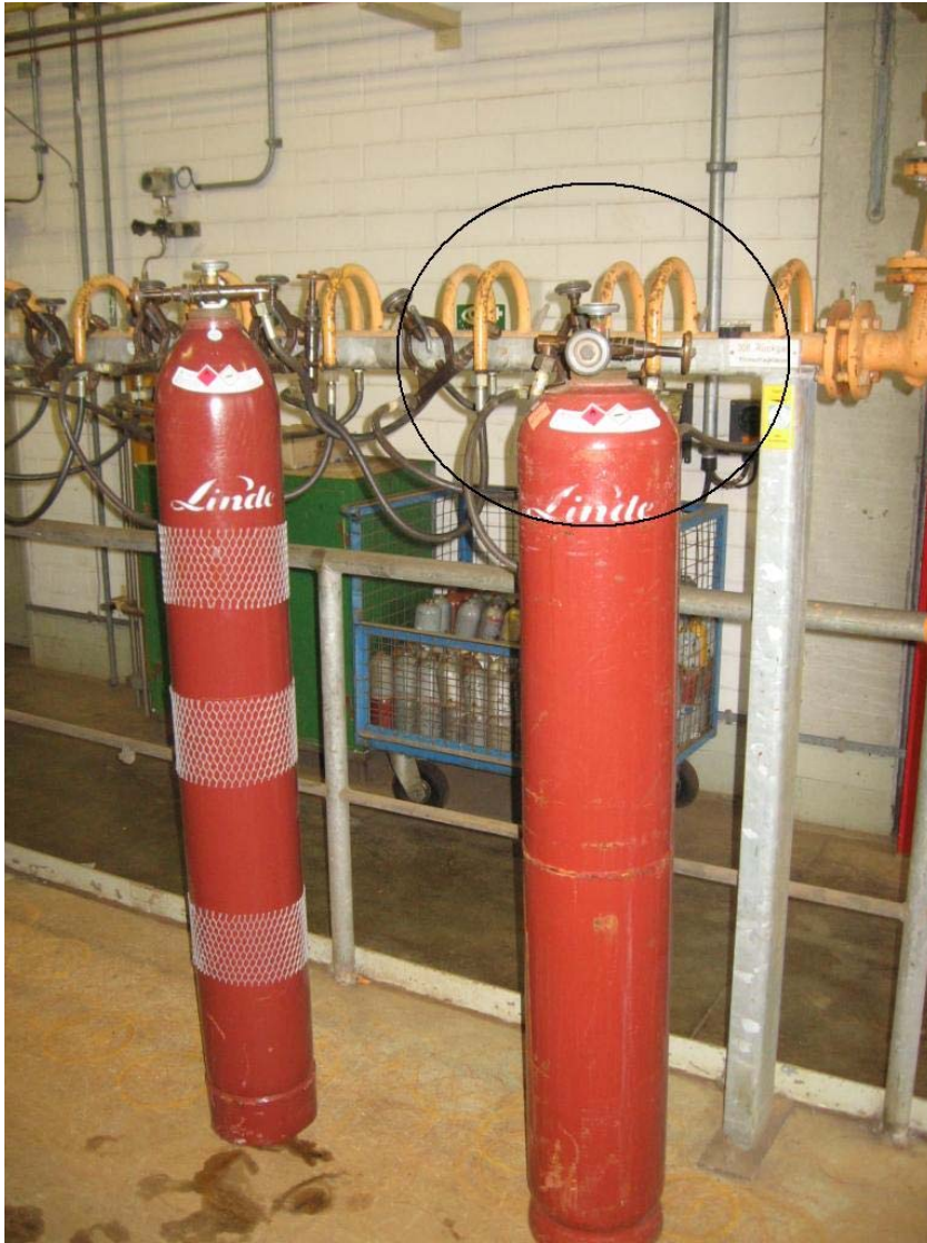
Figure 1: Emptying Cylinders in Production - Stop valve directly at cylinder (photo: Linde AG)
