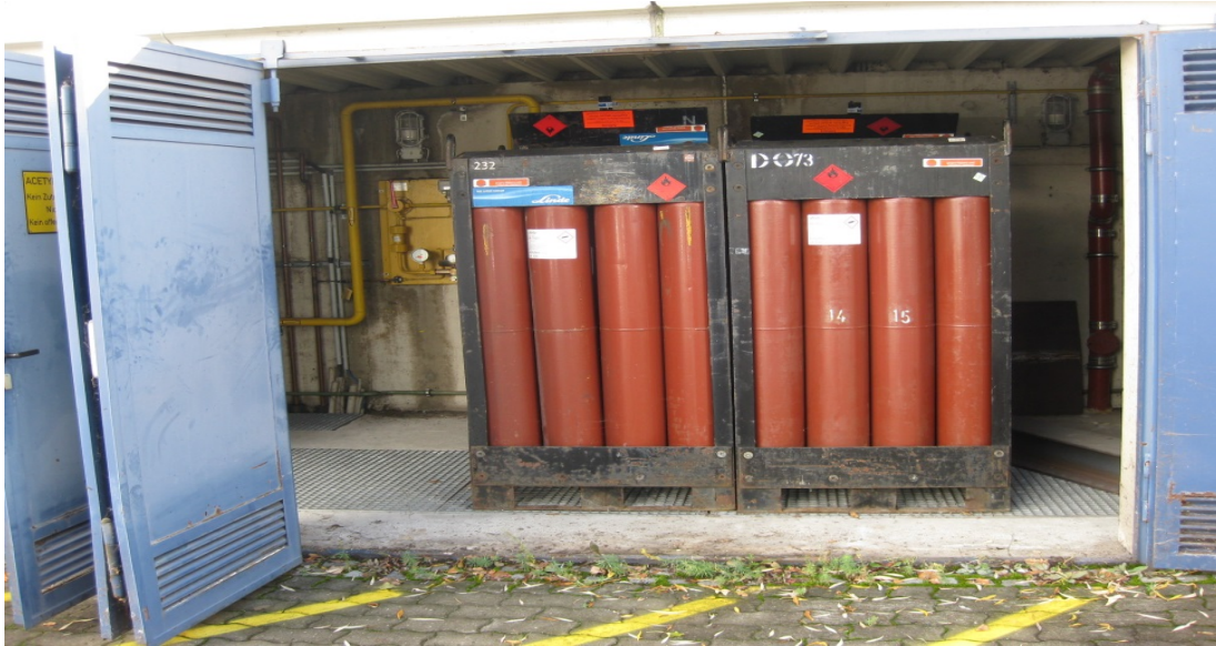
Figure 2: Customers supply system (photo: Linde AG)
