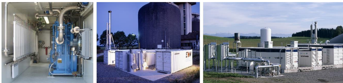
Figure 3: Three different membrane-based biogas upgrading plants (left: Bruck/Leitha in Austria ; mid: Wr. Neustadt in Austria; right: Kisslegg in Germany)
