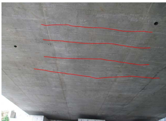
Figure 1: Transverse cracks on the bottom
