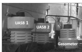
Figure 6: View of UASB System Biodigesters Plug Flow deployed in brewery in Jacareí SP Brazil.
