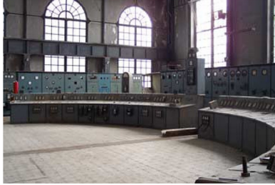
Fig. 4. Silahatara Electric Power Plant, 2nd Engine House
