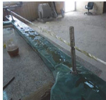
d) pulling out and twisting the fibers to squeeze out the excessive amount of the resin.
