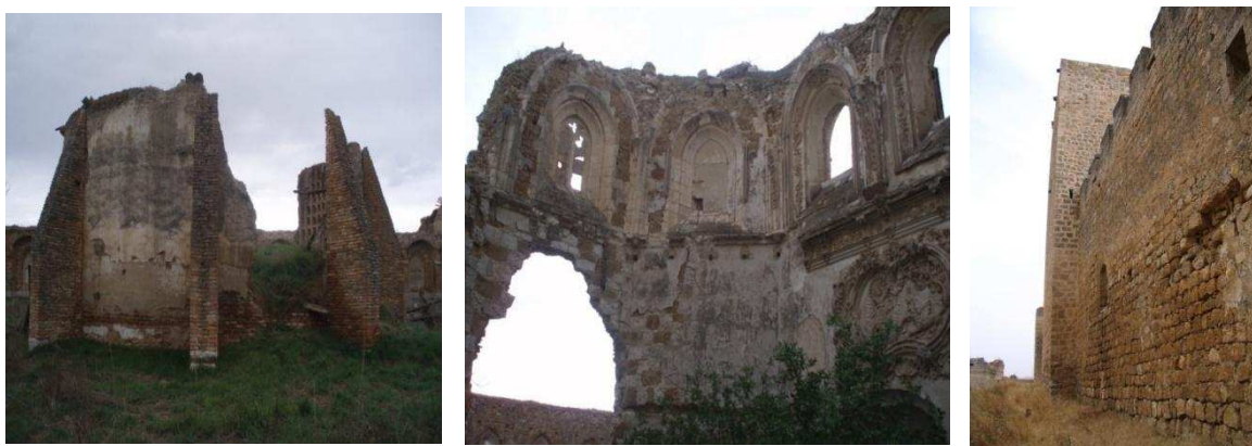
Figure 1: 1) Lack of verticality in walls of Chartres of Aniago (Valladolid, Spain). 2) Dangerous vaults in Aniago. 3) External walls in a Spanish Castle (Trigueros del Valle, Valladolid)
