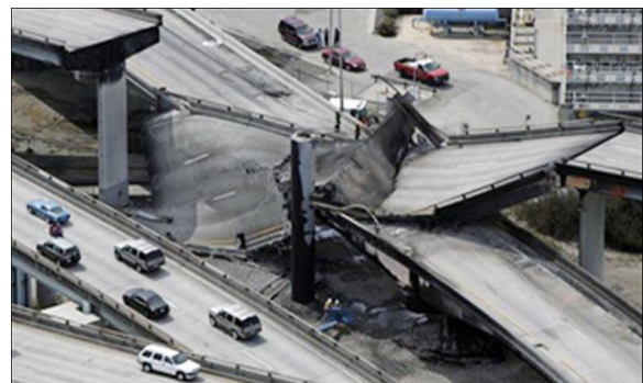
Figure 1. Oakland highway bridge collapse under fire due to gasoline tanker crashing, California, USA, 2007
