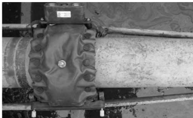
Fig. 4. An applied ring on a tube and two heating pipes that are bent out for application of the ring
