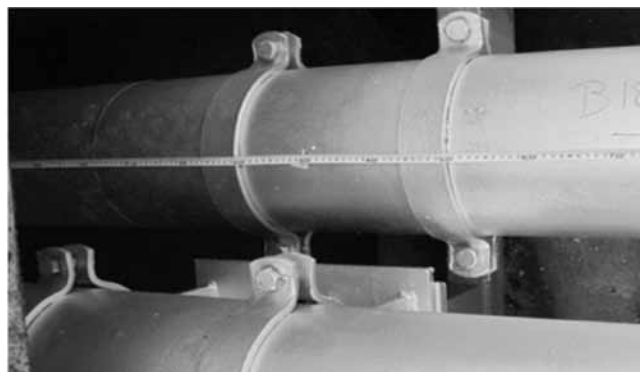
Fig. 5. Supportin clamps on the pipes
