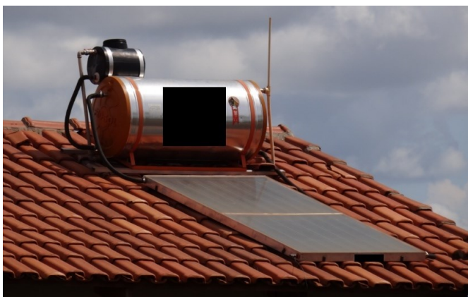
Fig. 1. Solar water heating system in home of low-income family
